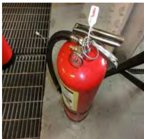
Figure 7: BullEx Smart Extinguisher filled and ready for use.
